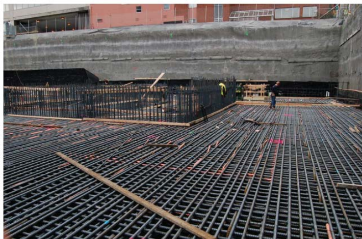
Figure 3–10. A newly published NIST Tech Brief presents advice for practicing engineers on designing mat foundations, such as this one under construction. © 2009 Image Courtesy of Magnusson Klemencic Associates.
