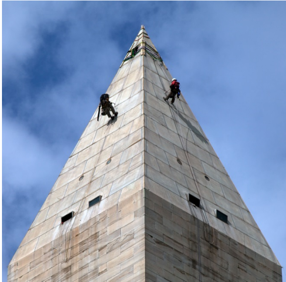
Figure 5–1. Engineers conducting an exterior assessment of the Washington Monument, which was damaged in the Mineral, VA, earthquake. Image courtesy of the National Park Service.
