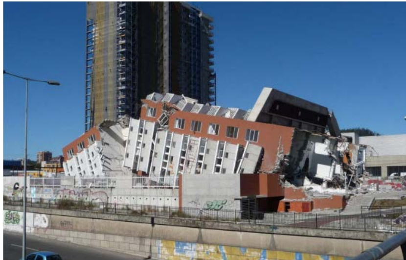
Figure 3–8. Collapse of the Alto Rio building in Concepción, Chile, in the 2010 Maule earthquake. A new report compares U.S. and Chilean design and construction practices so that U.S. engineers can learn from collapses such as this. Image courtesy of FEMA.
